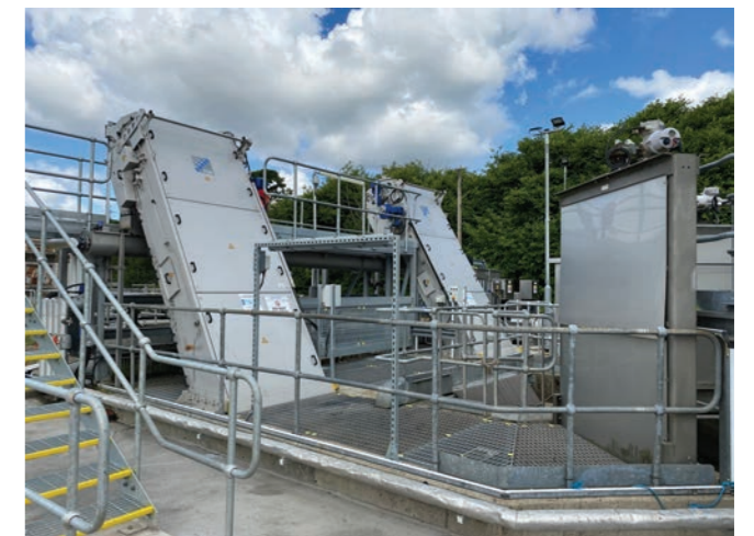
The new FSM FRS111 escalator screens installed at the Carbarns WwTW site, providing robust, and reliable screening.
