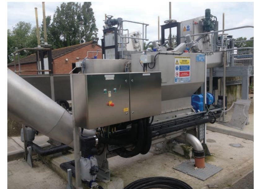
The Kuhn Wash Press transports, dewateres and compresses wastewater screenings.
