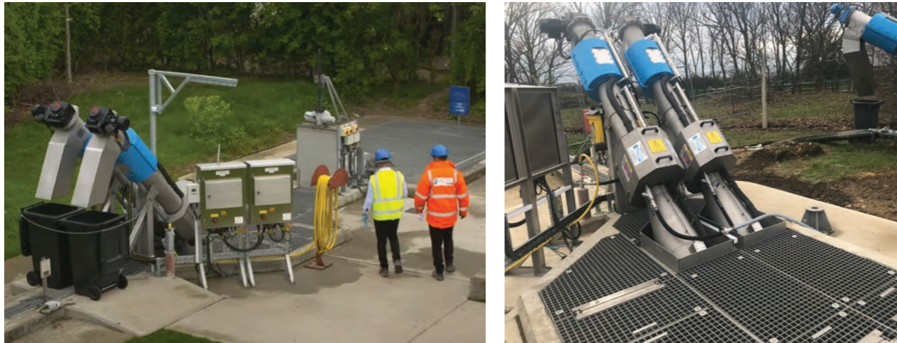
The MNSS Combined Screen inlet works package fitted directly into the existing channel, eliminating the need for costly civils works.
