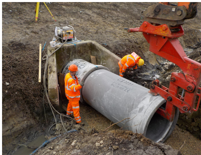
The project required dedicated stormwater treatment systems (Image © MJ Church)
