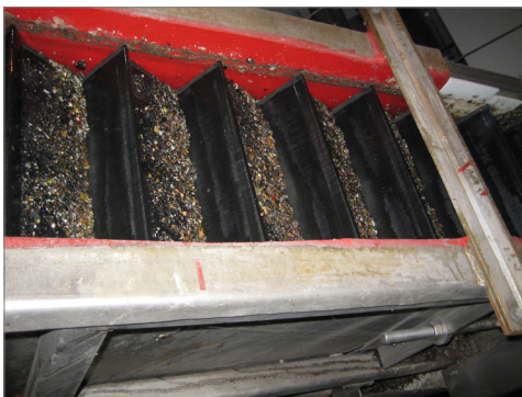
Grit and snail shells dewatered on Newton's Grit Snail® System
